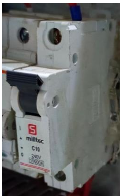
Fig.47. Image of HV cut-off switch
