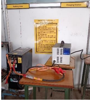
Fig.82. Charging station of battery pack
