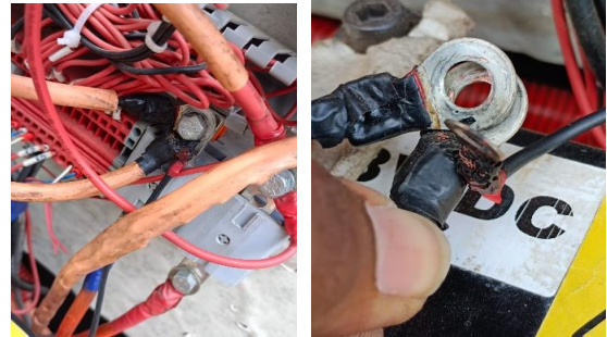
Fig.78. Wiring junction point melted because of vibration induces fastener loosening
