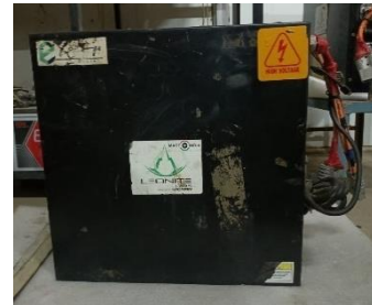
Fig.61. High voltage warning in motor, DC-DC converter, Battery pack
